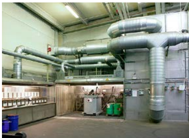
Filtration system and sorting stations
