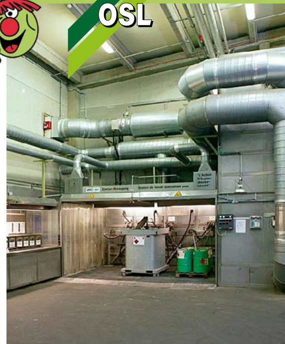
↑ Sorting and decanting station with a filtration system and continuous emissions monitoring
