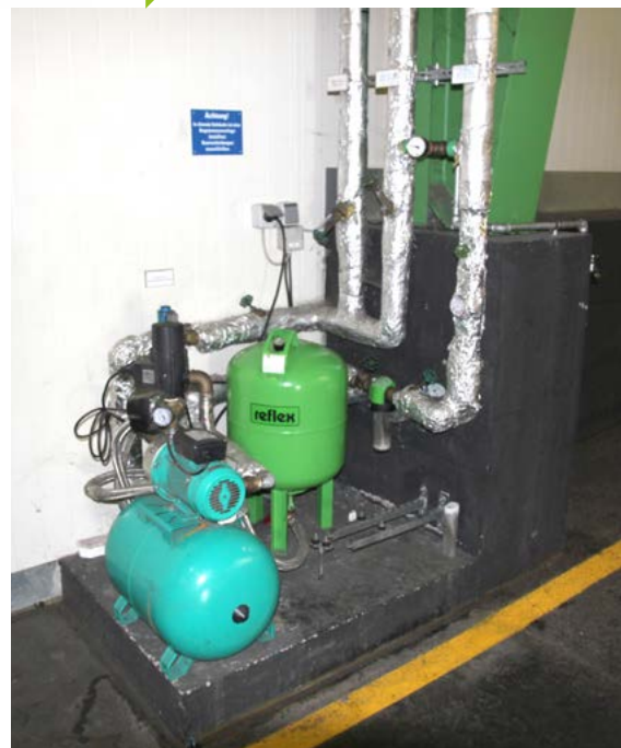
↑ Rainwater supply Rainwater savings are recorded via a separate water meter.
