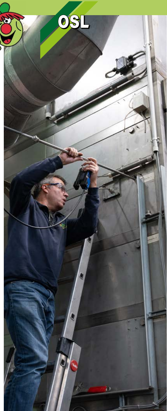
↑ Measurement at the filter tower
