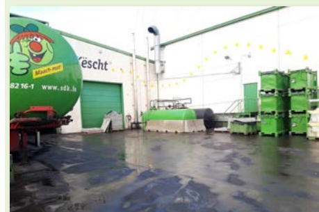
Washing area with oil and grease separator
