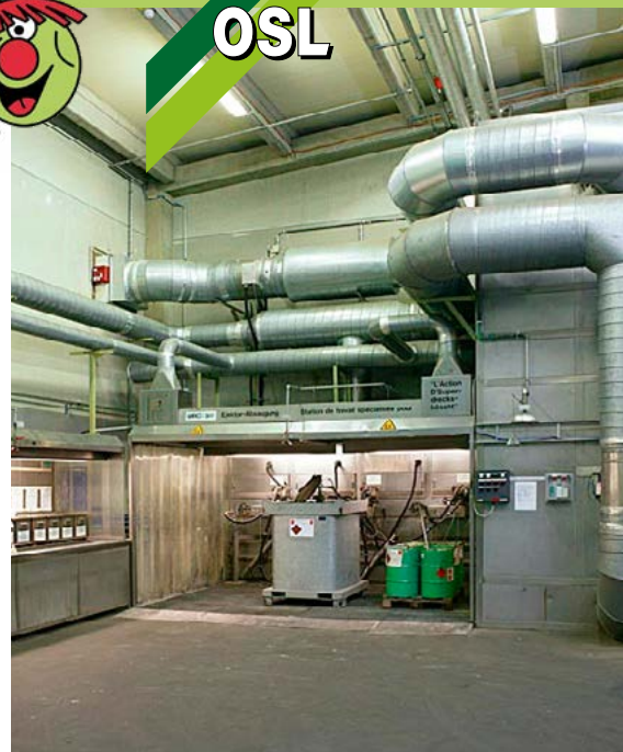
↑ Sorting and decanting station with a filtration system and continuous emissions monitoring
